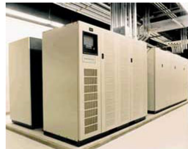
Centralized monolithic UPS
